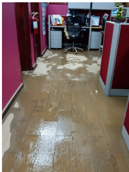
Remnants or evidence of flood inside Supercare Building
